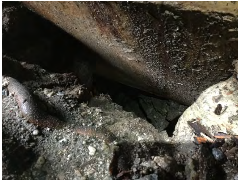
Scour under upstream left abutment lock block
