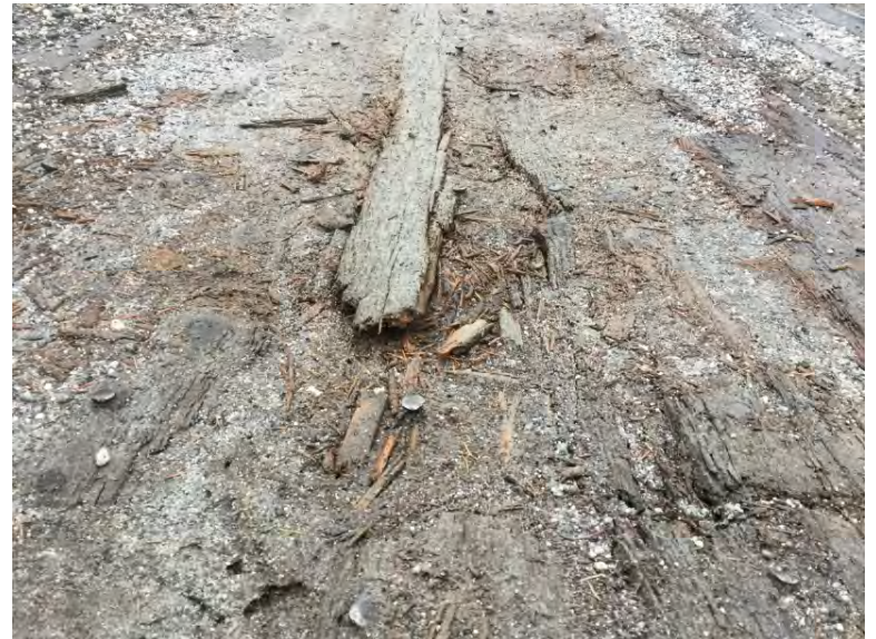
Nails protruding through planks
